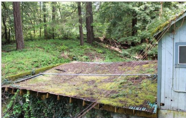
Roof deterioration and vegetation encroachment
