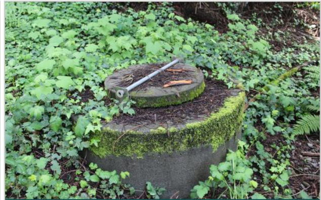
Small pump / manhole appurtenance
