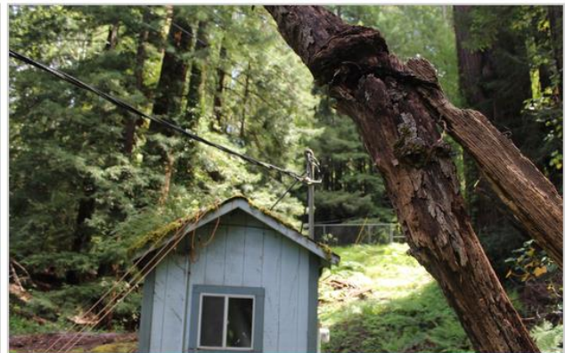
Tree / utility exposure upslope of structure
