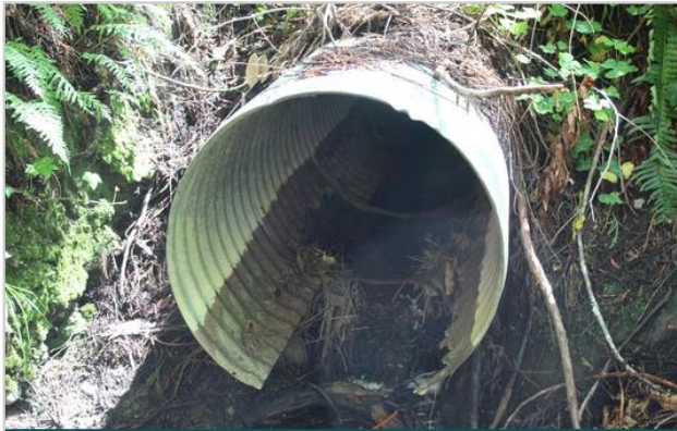
Damaged culvert outlet on spring property
